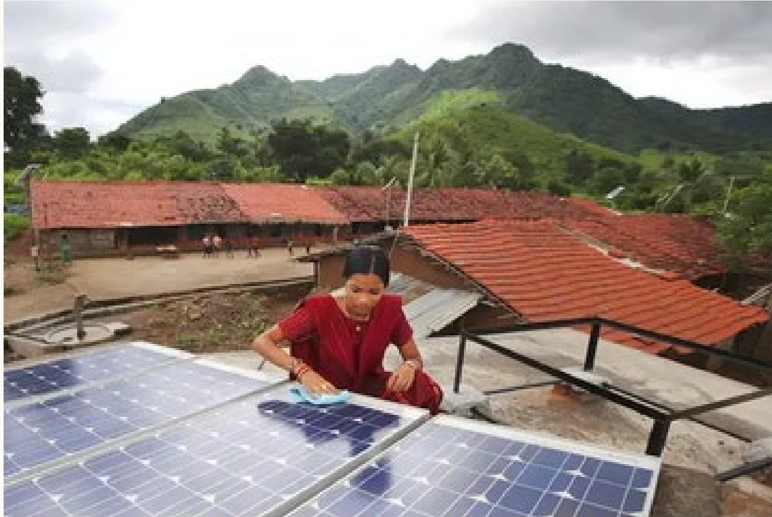
A solar installation in Tinginaput, India. ABBIE TRAYLER-SMITH / PAMOS PICTURES / DEPARTMENT FOR INTERNATIONAL DEVELOPMENT
